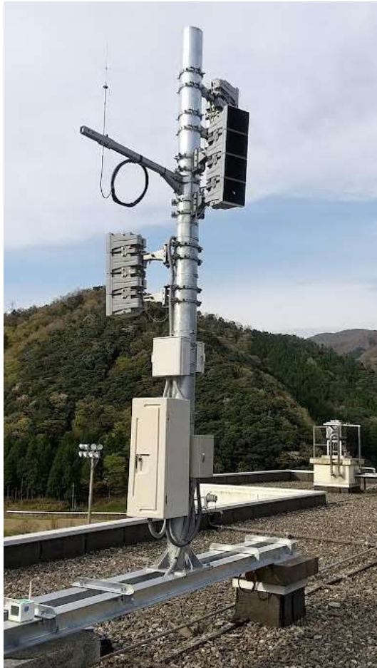
Disaster mitigation communication system Broadcasting device
